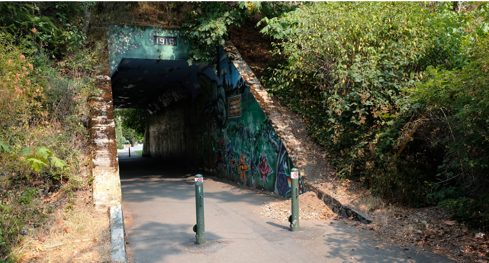
Atkins Road/Chilco Road Tunnel
